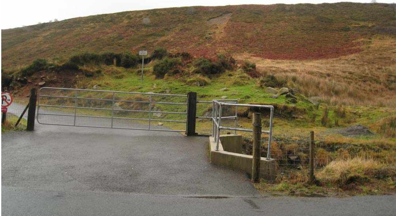
Fig PGGH_Dublin_004.3 Typical shallow slope failure in the Dublin Mountains
