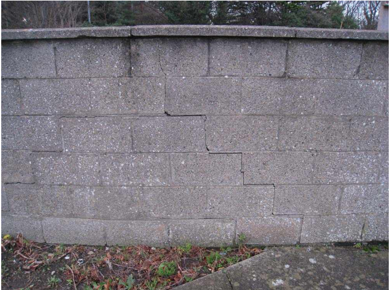
Fig PGGH_Dublin_003.4 Cracking in walls
