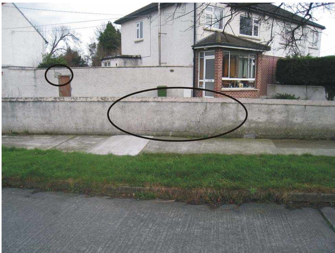
Fig PGGH_Dublin_001.8 Cracking in walls (circled)
