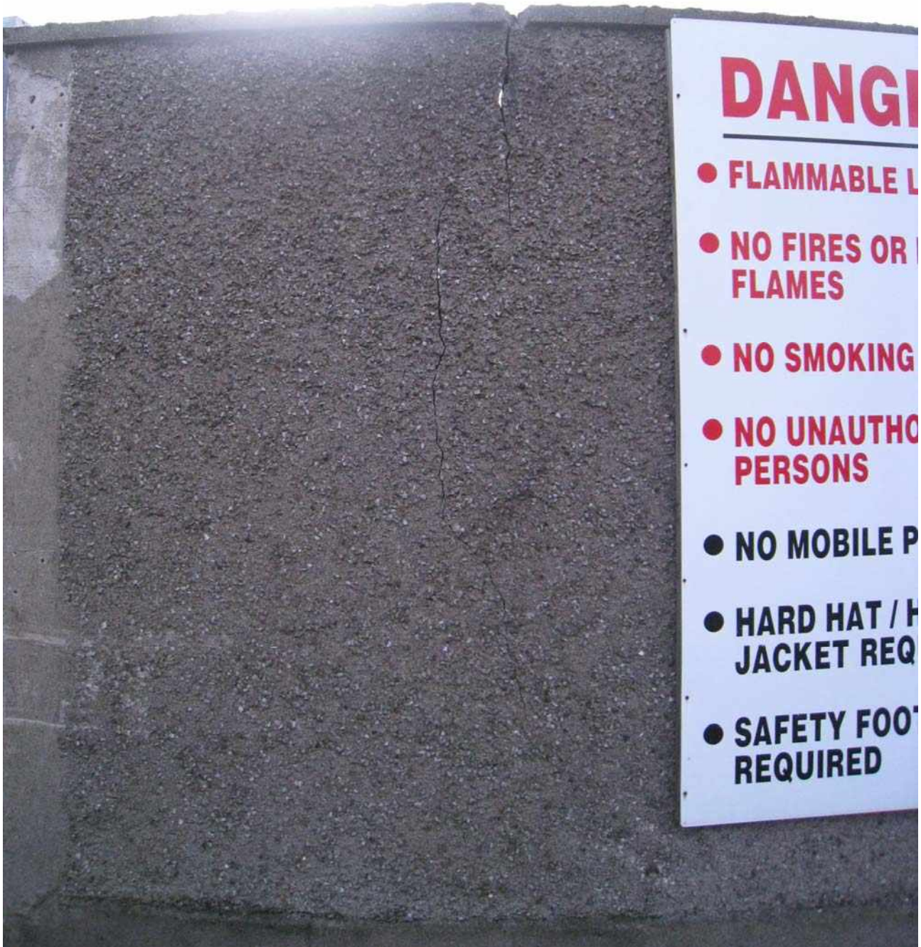
Fig PGGH_Dublin_006.4 Cracks in walls (clear daylight between)
