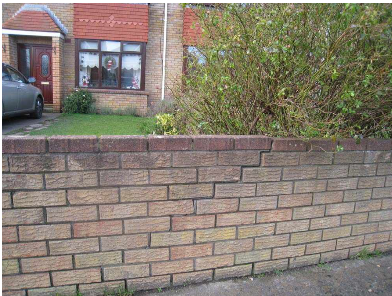
Fig PGGH_Dublin_001.7 Cracking in walls
