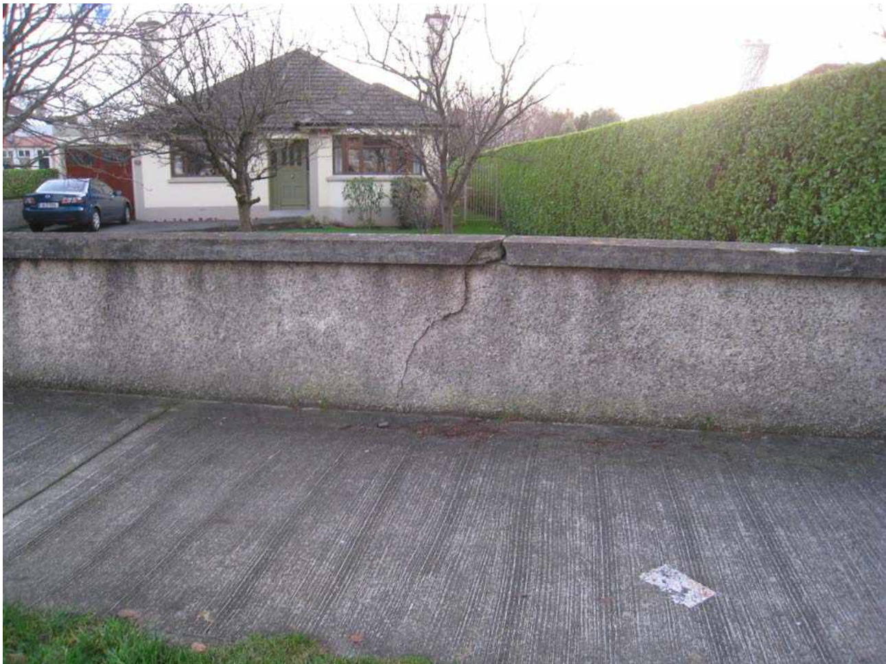
Fig PGGH_Dublin_003.2 Cracking in walls
