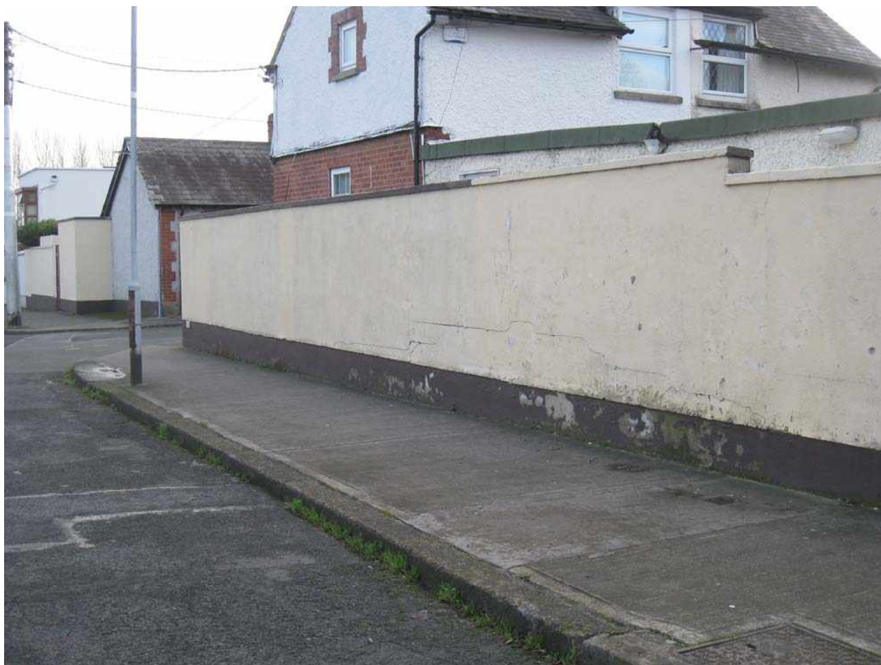
Fig PGGH_Dublin_006.8 Cracks in walls
