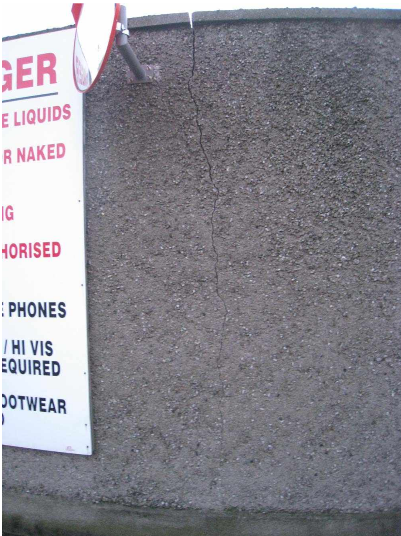
Fig PGGH_Dublin_006.3 Cracks in walls
