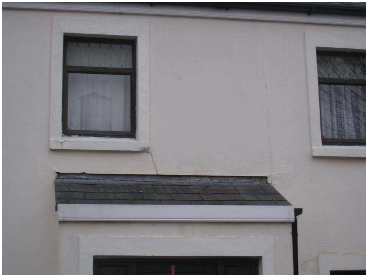
Fig PGGH_Dublin_006.6 Cracks in houses
