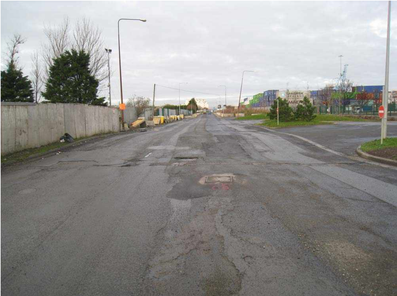
Fig PGGH_Dublin_002.3 undulations in a road surface and tilting lamp post
