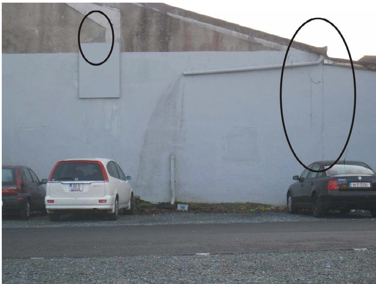
Fig PGGH_Dublin_001.5 Cracking in buildings
