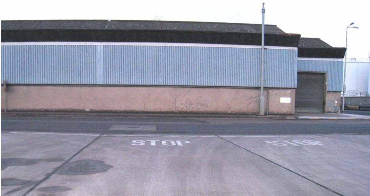
Fig PGGH_Dublin_006.2(a) Cracks in buildings
