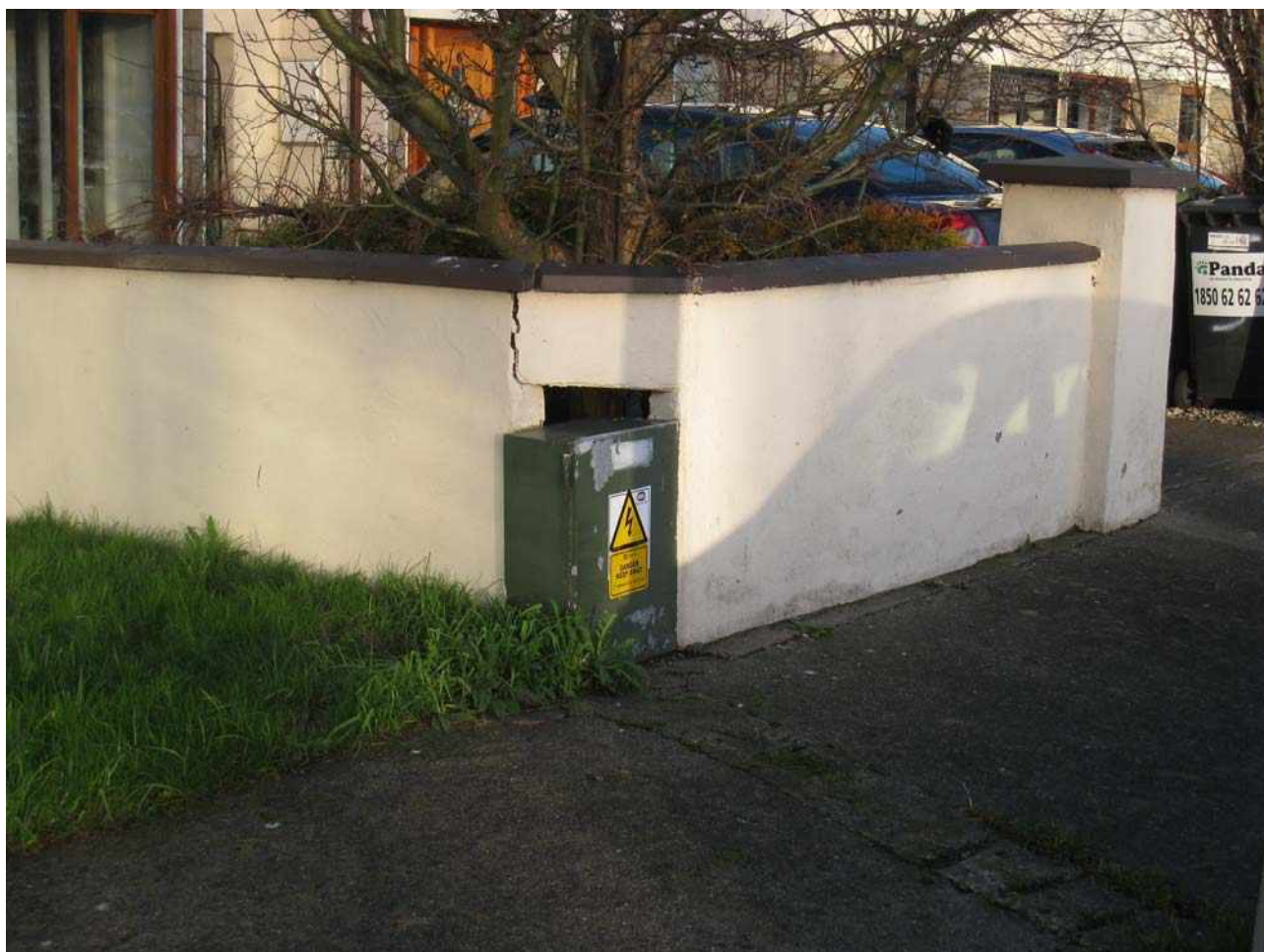
Fig PGGH_Dublin_008.7 Cracking in walls
