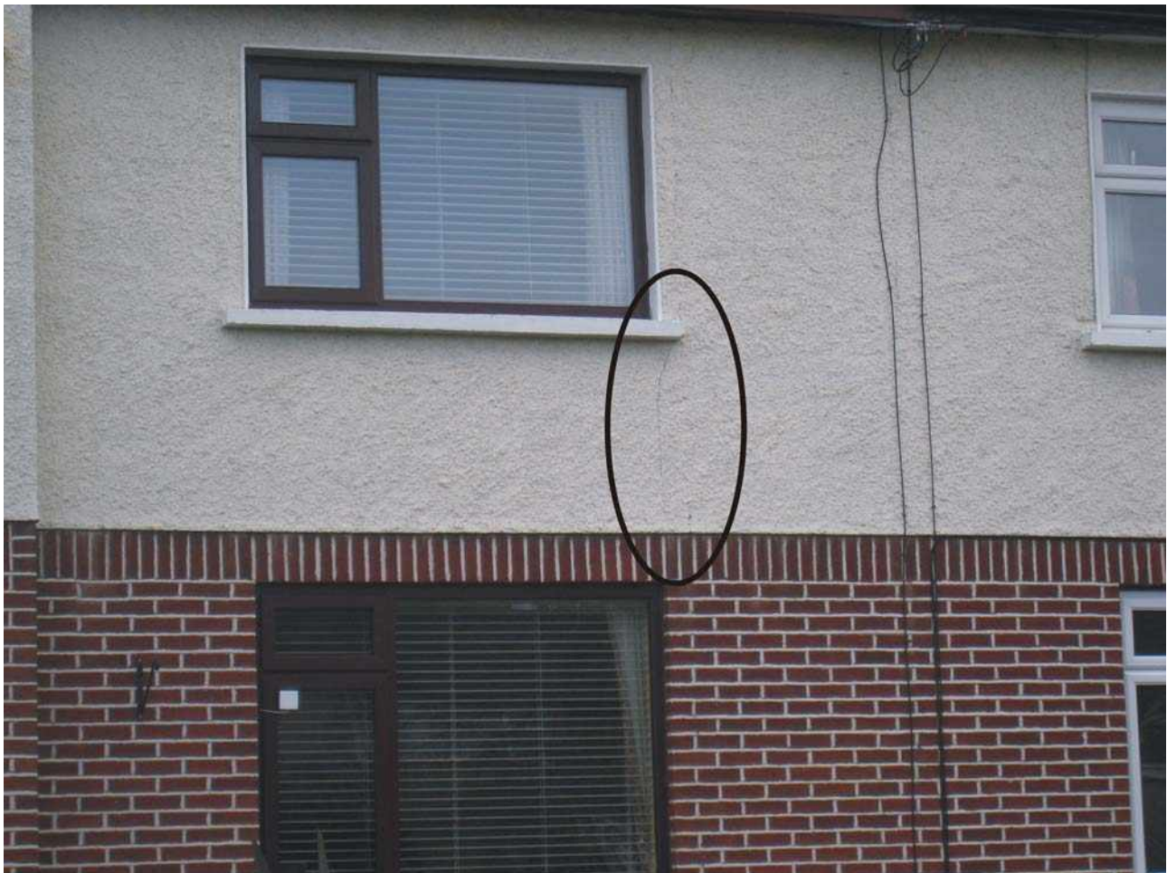
Fig PGGH_Dublin_001.9 Cracking in houses (circled)
