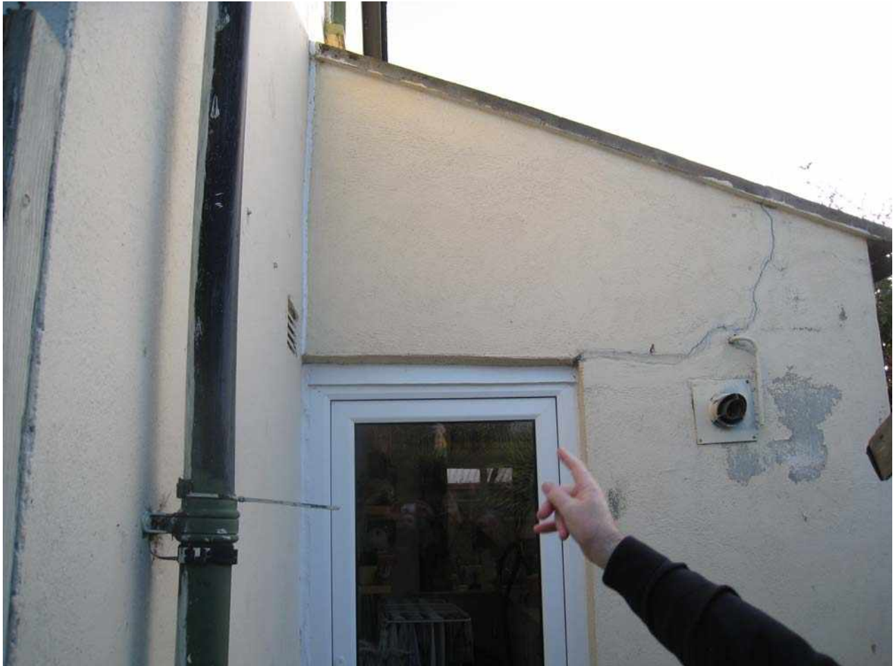
Fig PGGH_Dublin_008.10 Cracking in walls and differential settlement of building extensions
