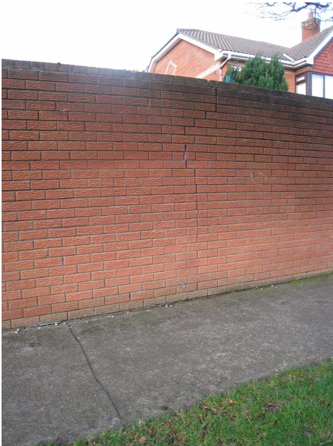
Fig PGGH_Dublin_001.6 Cracking in walls
