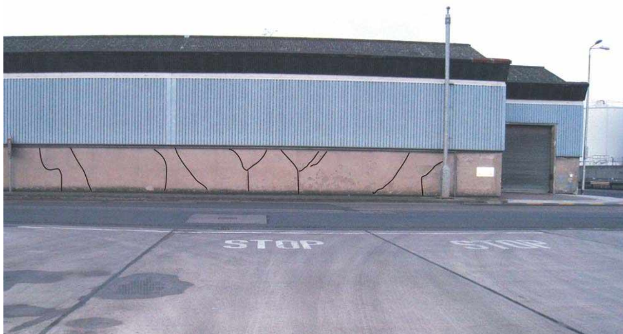
Fig PGGH_Dublin_006.2(b) Cracks in buildings highlighted
