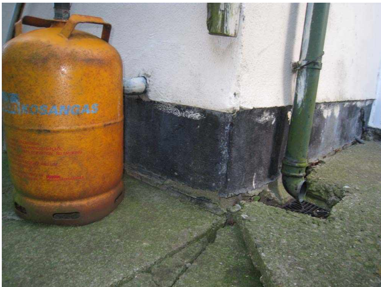
Fig PGGH_Dublin_008.8 Subsiding of paved areas
