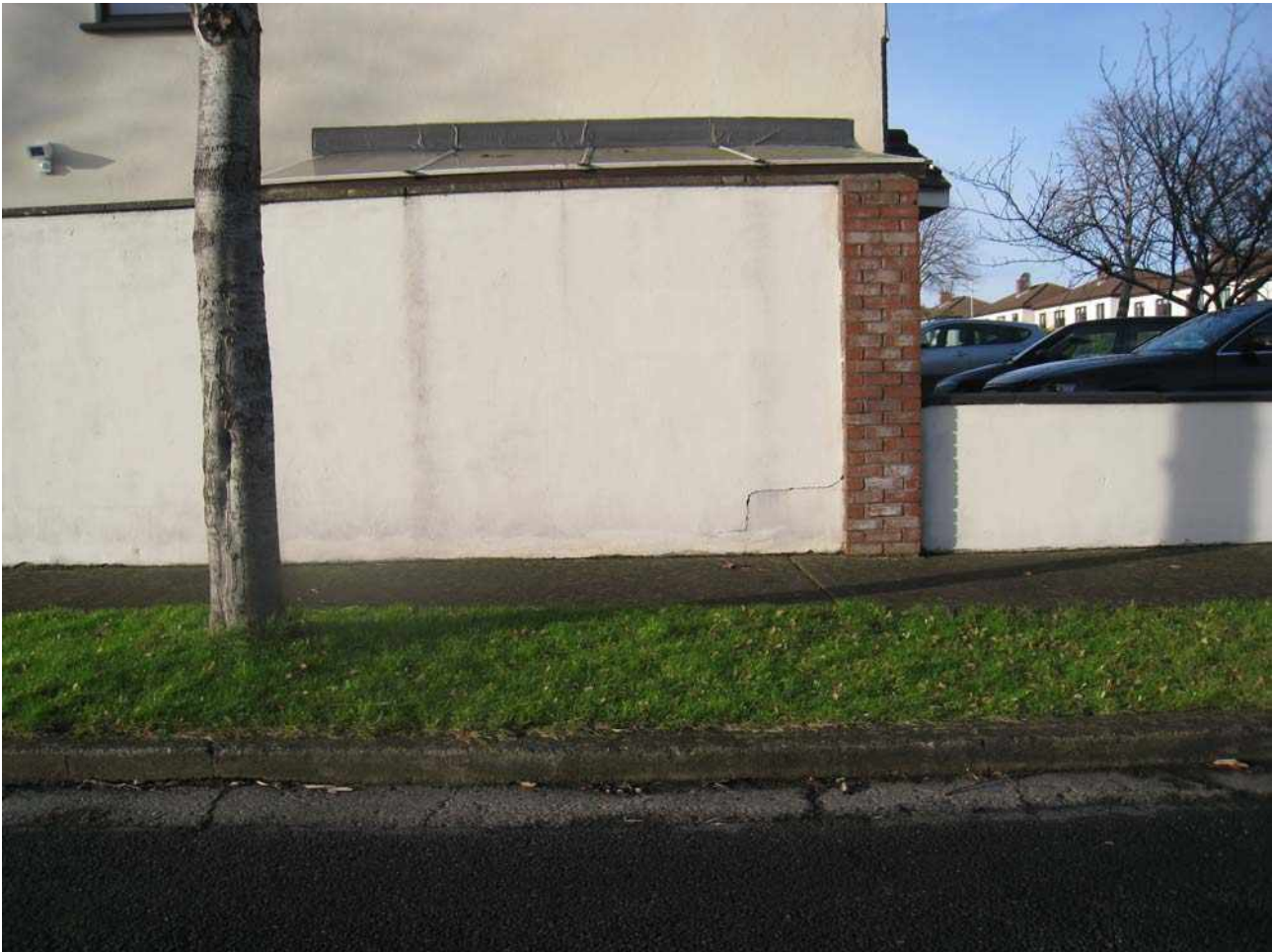
Fig PGGH_Dublin_001.3 Cracking in walls
