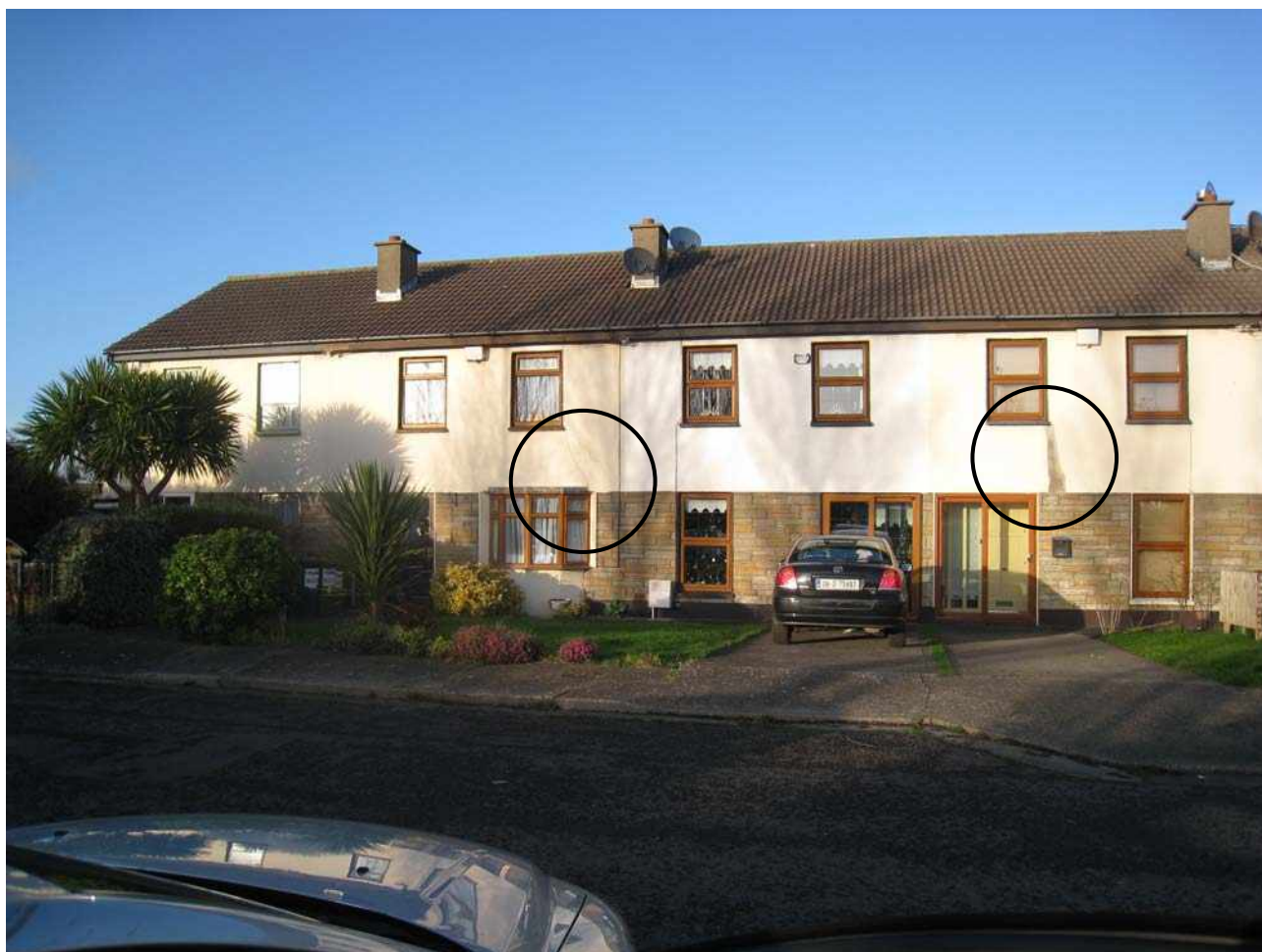
Fig PGGH_Dublin_008.6 Cracking in buildings (circled)
