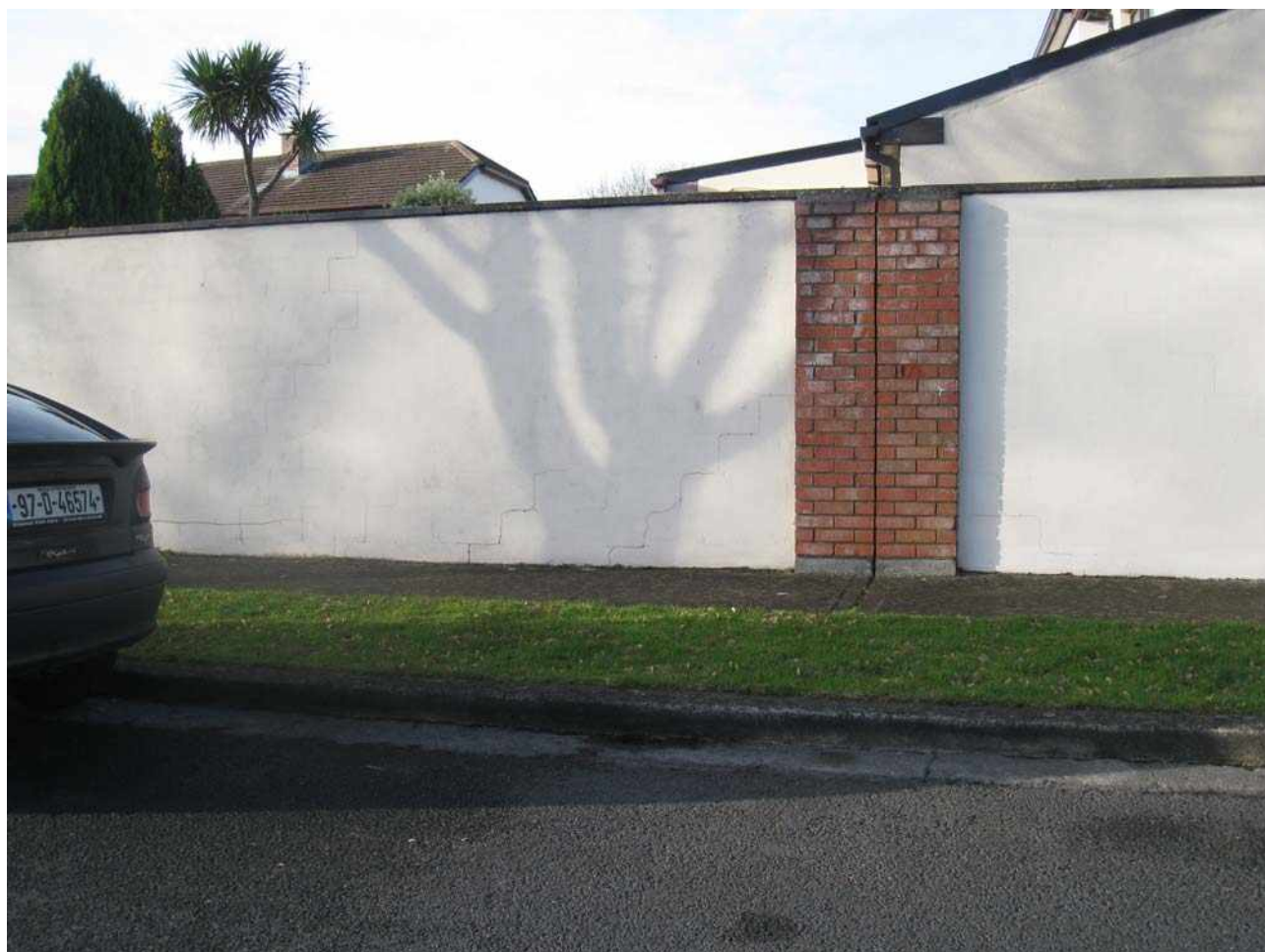
Fig PGGH_Dublin_001.4 Cracking in walls
