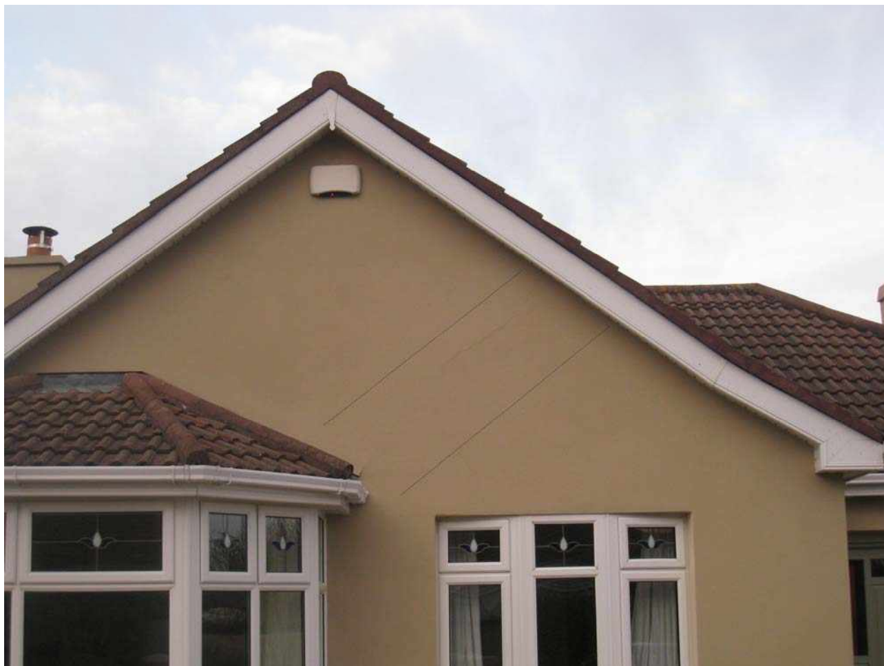
Fig PGGH_Dublin_003.3 Cracking in houses (within the lines)
