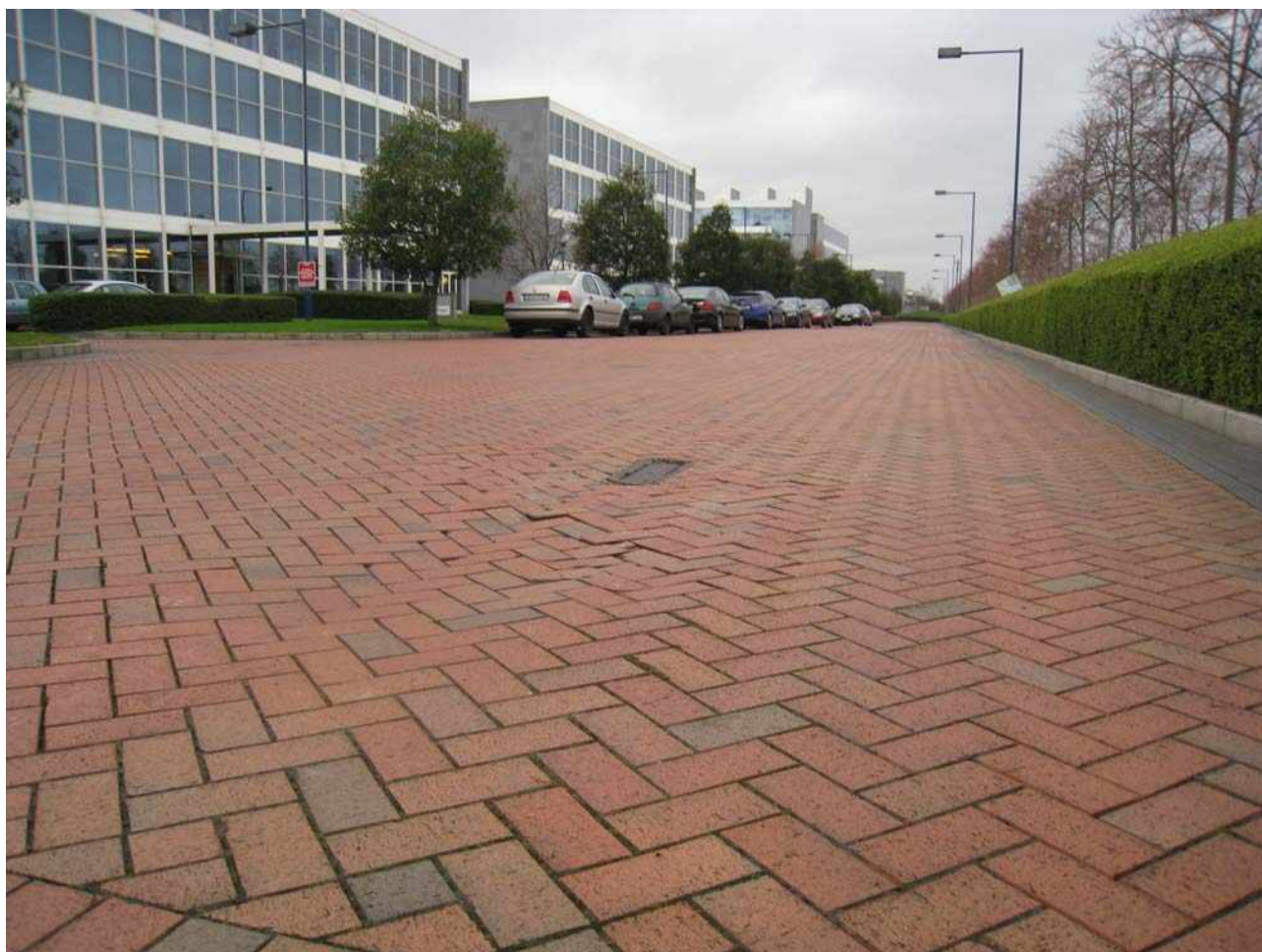
Fig PGGH_Dublin_006.5 Undulations in pavements
