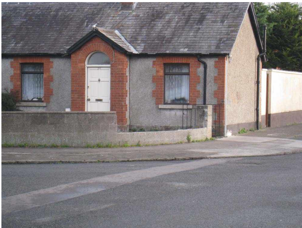
Fig PGGH_Dublin_006.9 Wall collapse
