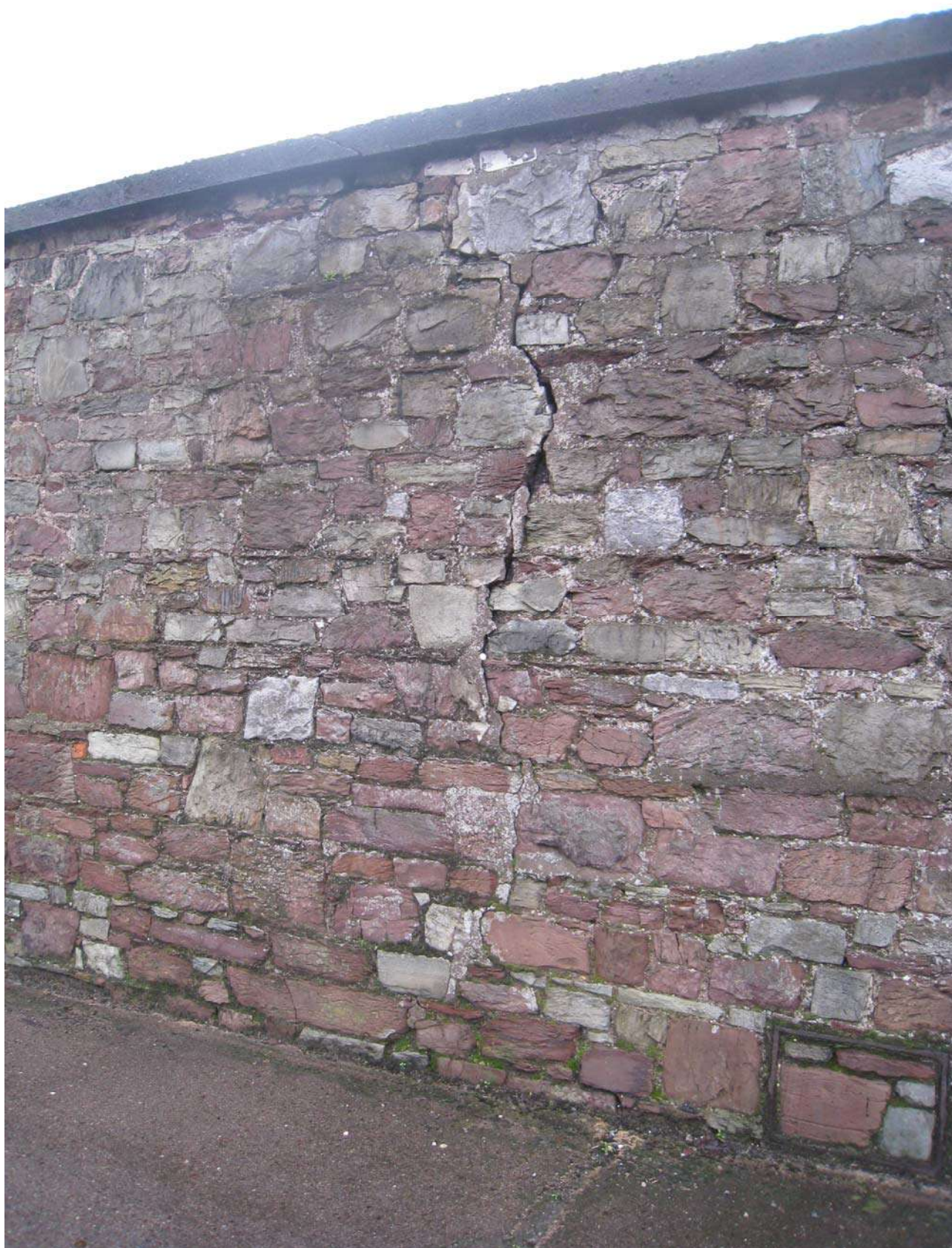
Fig PGGH_Cork_001.5 Somewhat repaired crack in a 3m high wall
