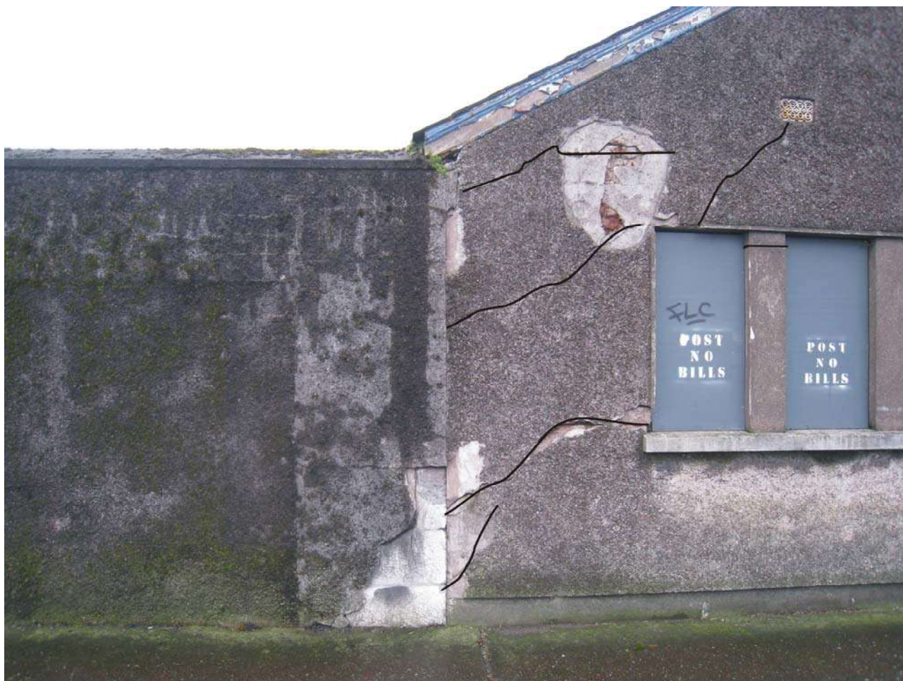
Fig PGGH_Cork_001.4 Cracks in building (highlighted)
