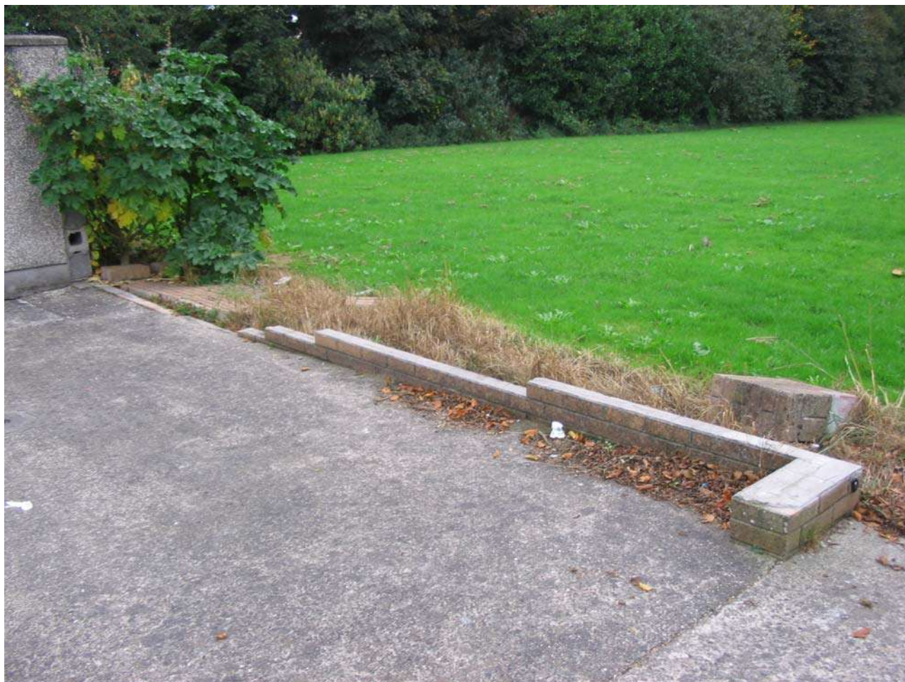
Fig PGGH_Cork_004.7 Collapsed walls
