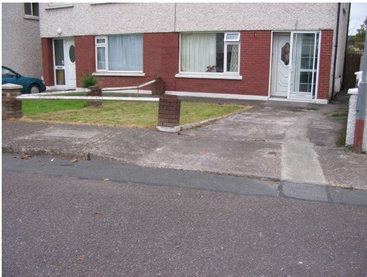
Fig PGGH_Cork_004.9 Subsidence of paved areas and tilting of structures
