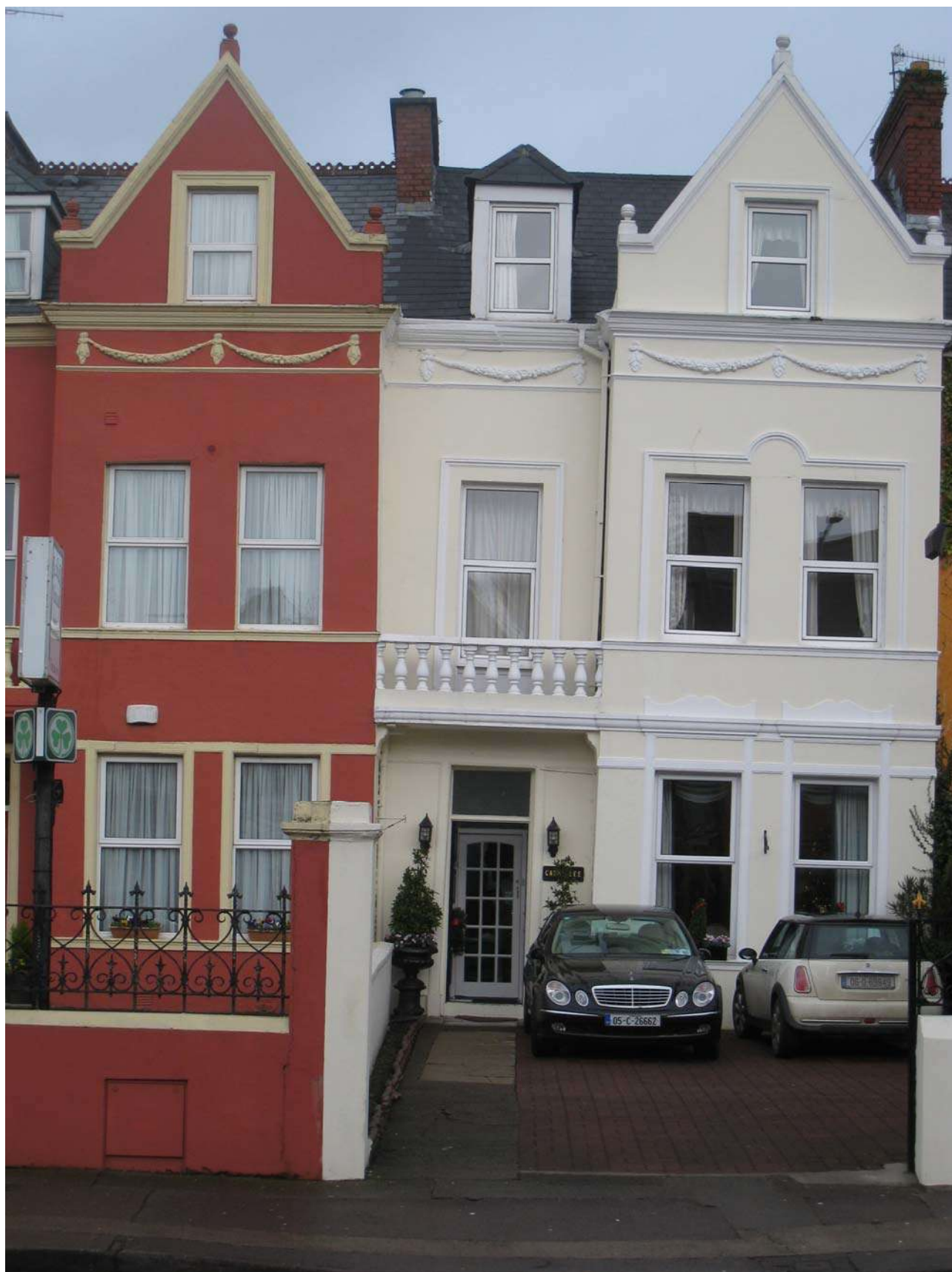
Fig PGGH_Cork_004.4 Tilt in buildings
