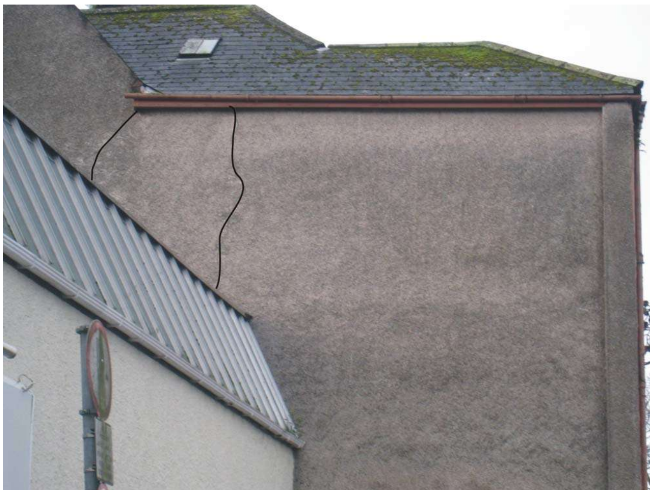
Fig PGGH_Cork_001.6 Cracks in building (highlighted)
