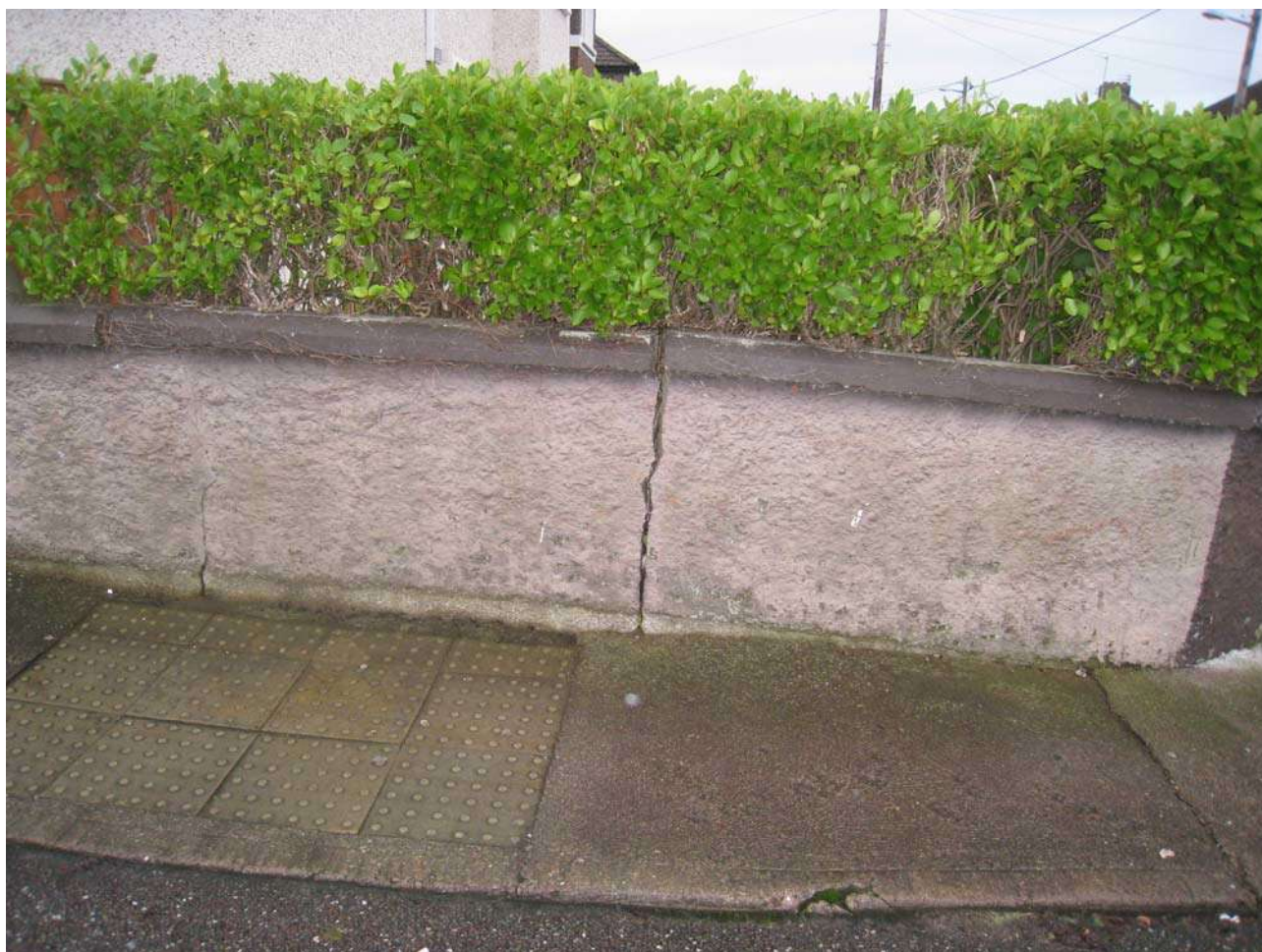
Fig PGGH_Cork_002.6 Cracking and displacement in walls
