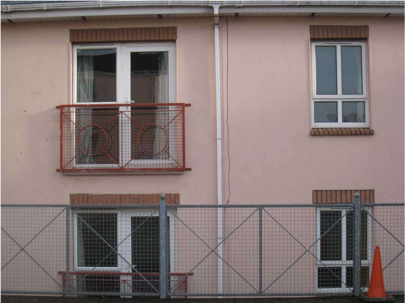
Fig PGGH_Cork_001.3 Cracks in building and slight tilting
