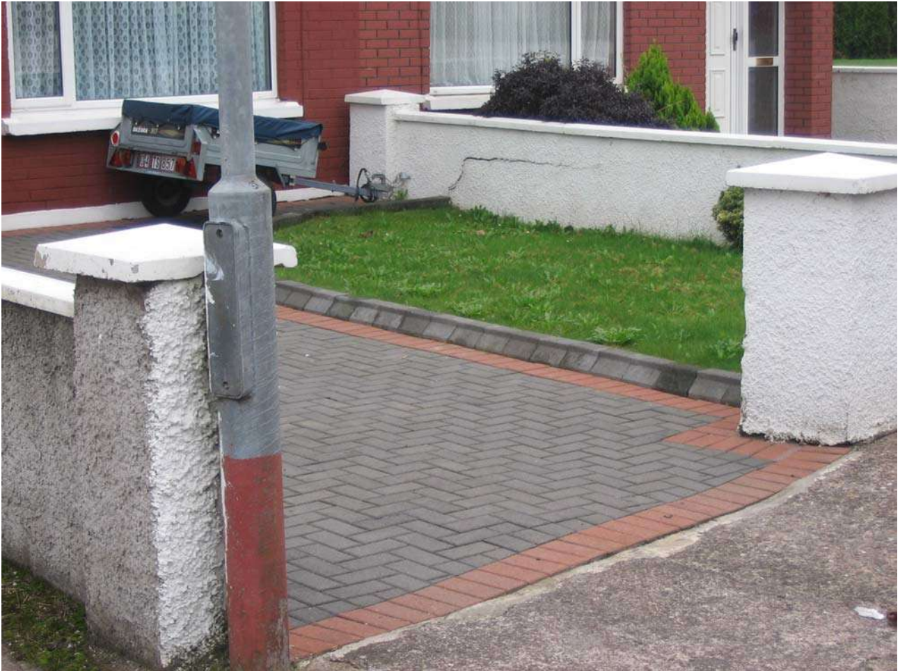
Fig PGGH_Cork_004.10 Recent underpinning and cracked walls
