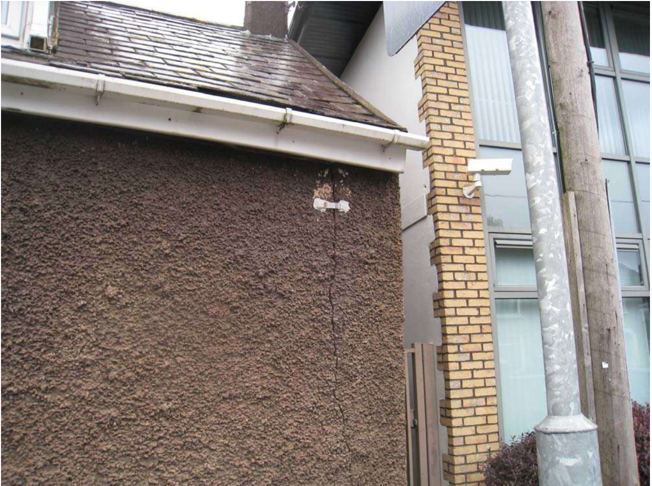
Fig PGGH_Cork_002.4 Cracking in building
