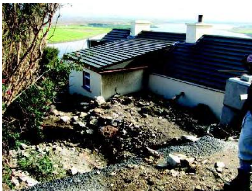
Plate 6.1 Damaged House at Pollatomish
