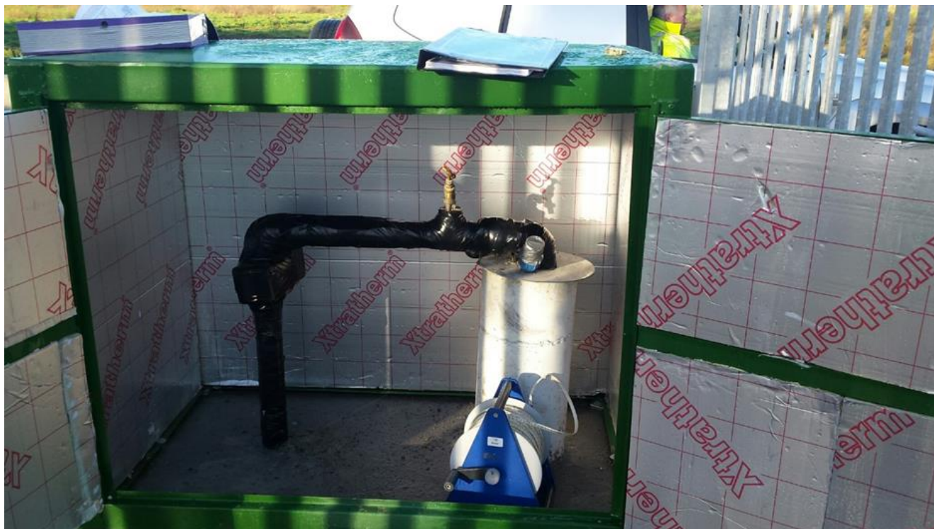
Photo 1: Example of good wellhead protection
