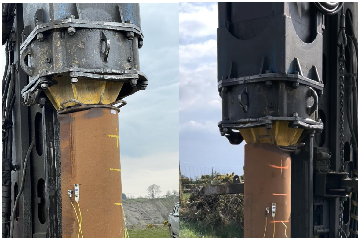
Figure 11: Damage to pile head for (a) Pile L3 and (b) Pile L4 in Blessington
