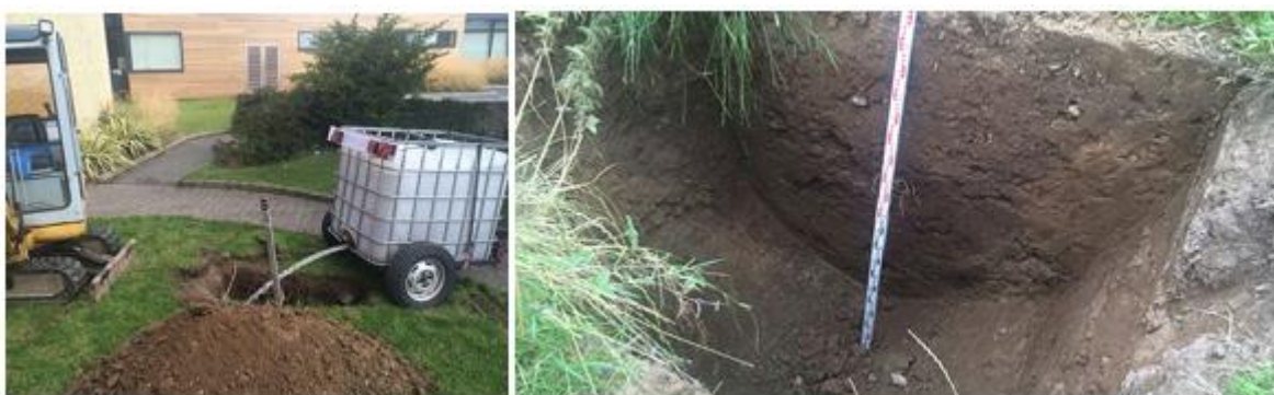
Figure 34 Percolation test ( http://www.percolationtests.ie/ ).
